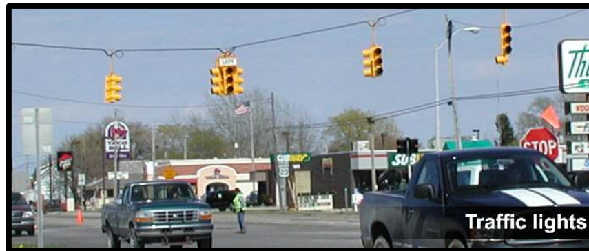
Figure D-1: Example of traffic signals
