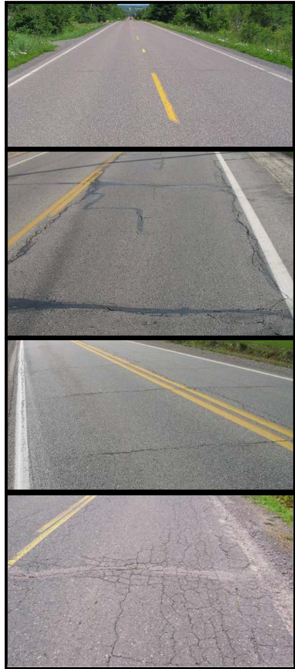
Figure 1: Top image, right – PASER 8 road that is considered “good” by the TAMC exhibit only minor defects. Second image, right – PASER 5 road that is considered “fair” by the TAMC. Exhibiting structural soundness but could benefit from CPM. Third image, right – PASER 6 road that is considered “fair” by the TAMC. Bottom image, right – PASER 2 road that is considered “poor” by the TAMC exhibiting significant structural distress.
